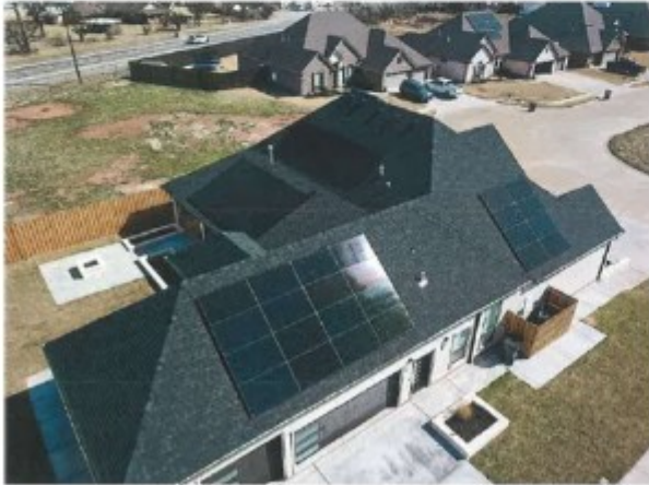
This is a typical roof mounted solar array.
