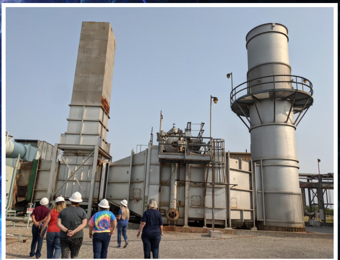
Jet engine housing, boilers, steam stack.
